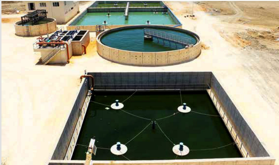
Biological and chemical treatment tanks
